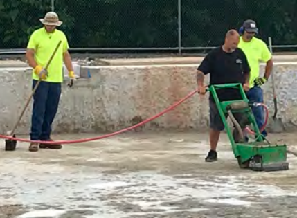
Roughing up the surface to pour a new concrete surface. Pool is targeted to be opened by the second week of July.
