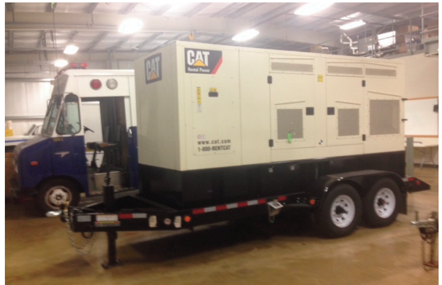
Caterpillar trailer-mounted 200 kW emergency generator will be transported to VFW Post 2290 on Washington Avenue if future emergency sheltering is needed in Manville.
