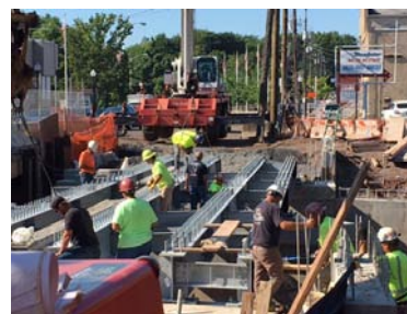
South Main Street bridge project progress continues on schedule to meet the completion date in August 2018.
